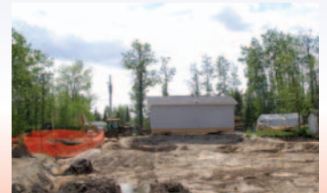
Fuel Spill at Remi Lake in Moonbeam. D&G Construction's specialized spill response team remediated seven properties. The remediation consisted of soil removal, boathouse reconstructions and landscaping.
